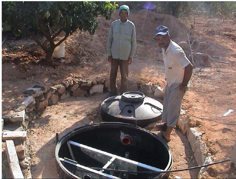
Photo (6): Small Waste Water Treatment Plant
