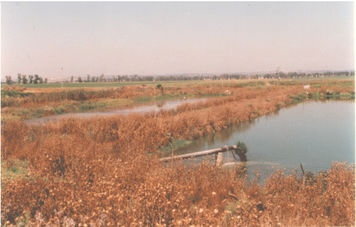
Photo 1: Wastewater Treatment Plant for Tulkarm City
