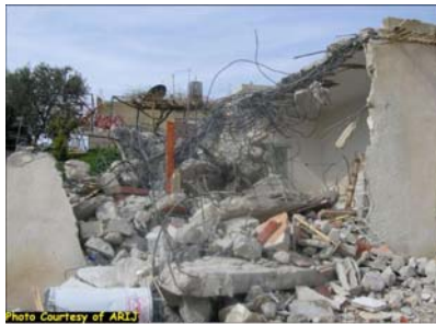
Photo Courtesy of ARIJ The demolished house of Khader Dar'awi
