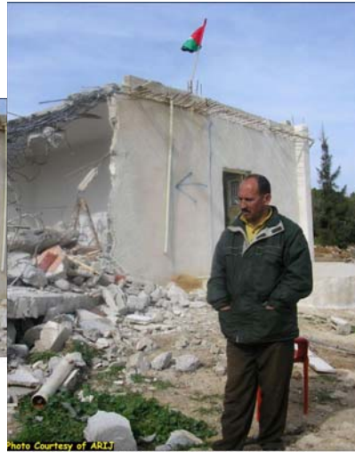
Photo Courtesy of ARIJ Mr. Nidal Dar'awi standing in front of his brother's demolished house.
