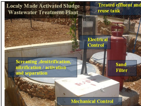
Figure 2: Description of the different components of a locally made onsite wastewater treatment system (ARIJ, 2005).
