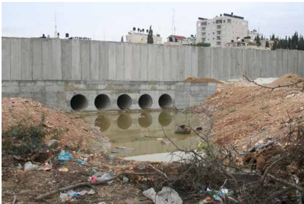
Picture 1: Wastewater in Ar Ram
