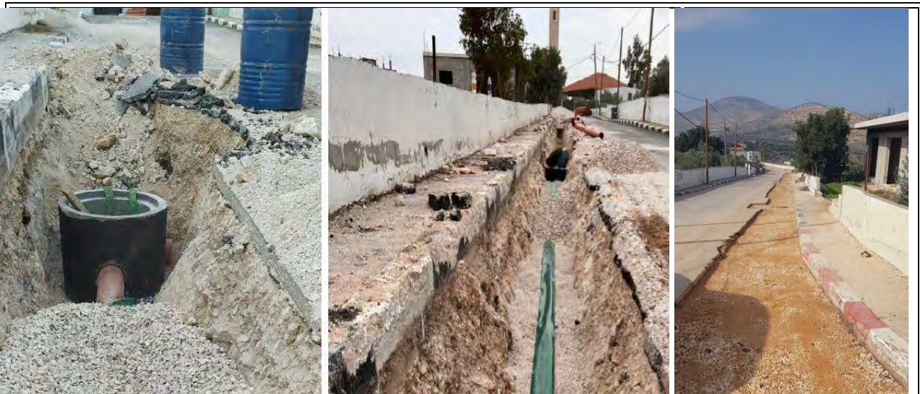
Figure 3: The constructed of the sewage network and household connection at Al Aqaba- Tubas
